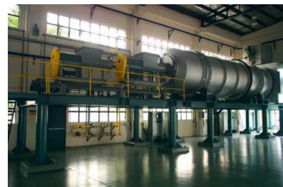
Figure 4. Rotary Kiln Gasifiers
